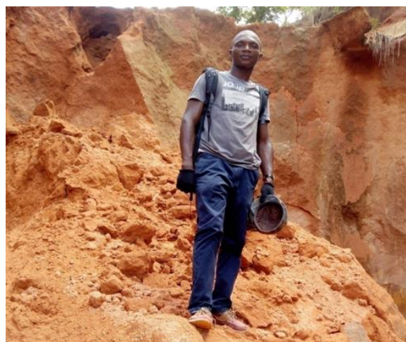
Plate 1: Gully resulting from failed road construction in Amainyi Ihitte Uboma in UIRB in 2019
